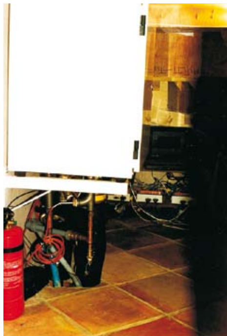
Figure 6 The heat pump was installed in an understairs cupboard
