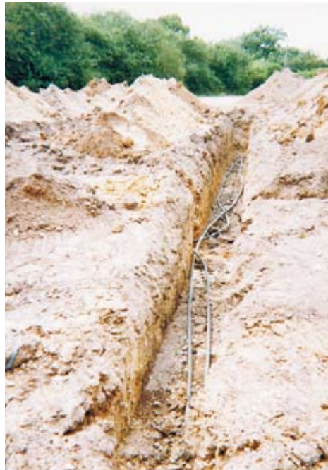
Figure 5 200m of ground coil was used at an average depth of 1m
